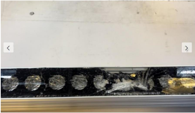
The glass surface cover is completely broken
